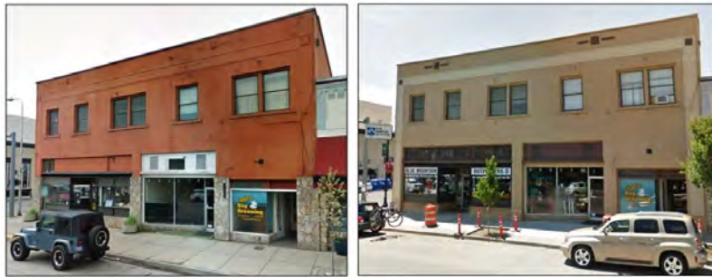
Ralston Block (1124 Adams Avenue) Note the removal of the added “fieldstone” facing and restoration of the historic painted brick wall finish. (Source: Google Street View 2012 and 2015)
