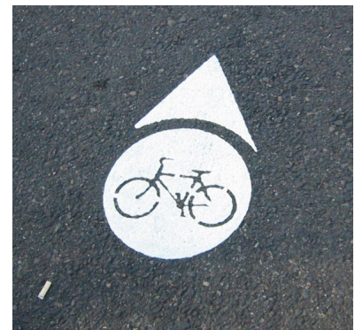
Figure 5-13. Directional pavement marking
