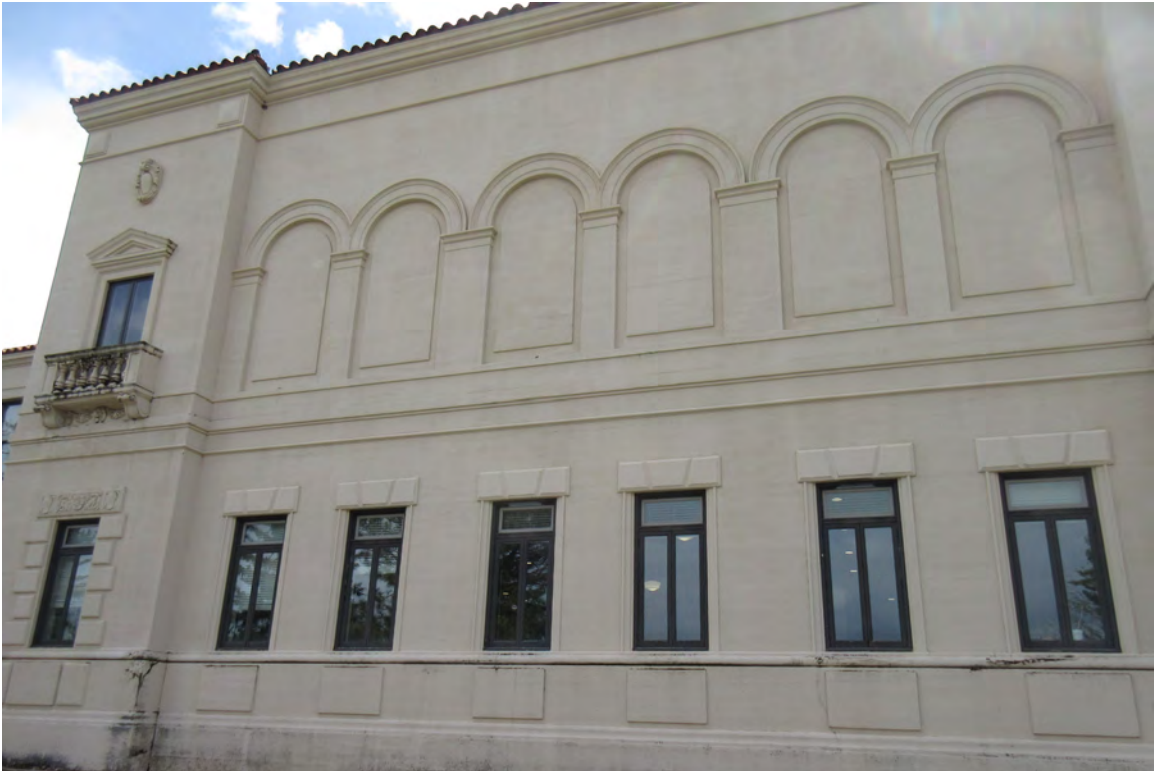
9. Central pavilion, north elevation. The concrete detailing in the archways will be replaced with windows that match the windows of the south elevation second floor, facing south. 04/19/2022.
