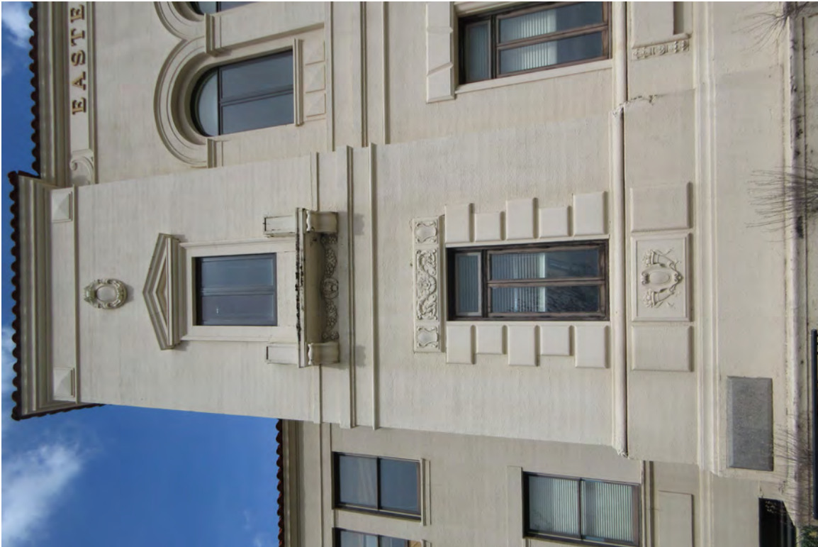
7. Inlow Hall south elevation, facing north. Notice damaged Juliet balcony. Juliet balconies are either damaged or missing on both north and south elevations. 04/19/2022.
