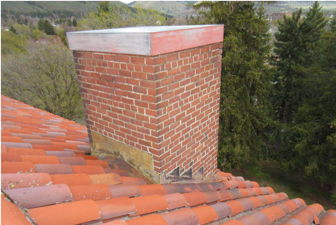
12. Inlow Hall's chimney to be removed and replaced with terracotta roof tiling on the north side of the west wing, facing northwest. 04/19/2022.
