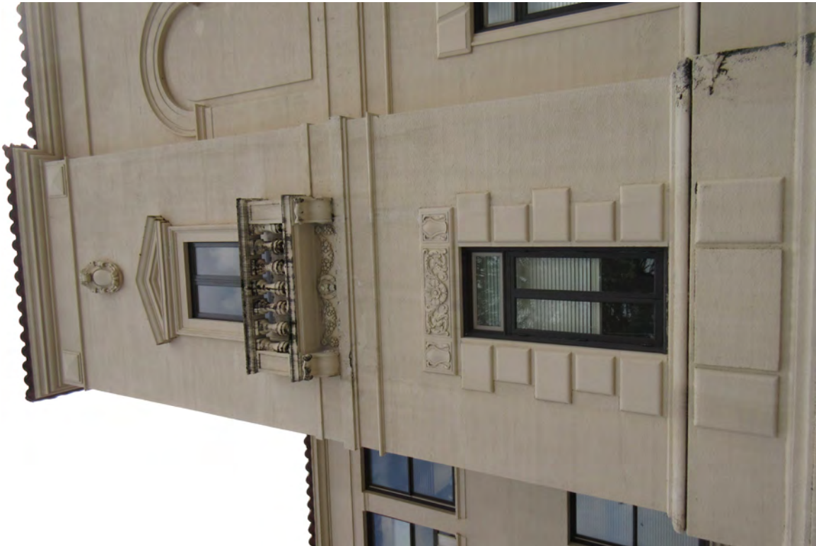
8. Inlow Hall north elevation, facing south. Notice deteriorating Juliet balcony. 04/19/2022.
