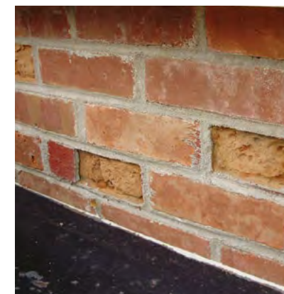
[2] Not Recommended: The use of inappropriate Portland cement mortar to repoint these soft 19th-century bricks has caused some of them to spall. Photo: Courtesy Nebraska State Historic Preservation Office.
