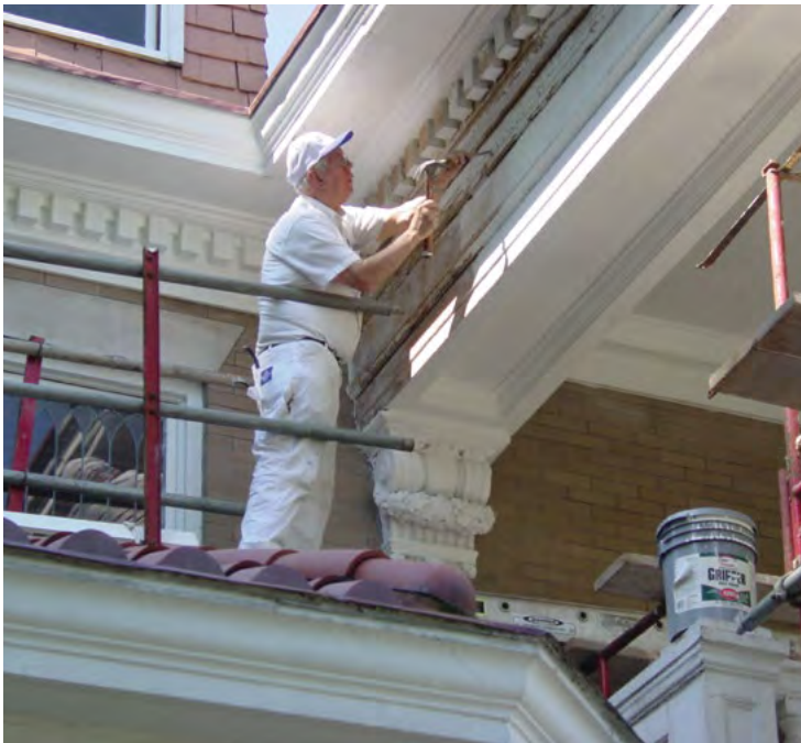
[12] Repair and limited replacement in kind to match deteriorated wood porch features is always a recommended preservation treatment.
