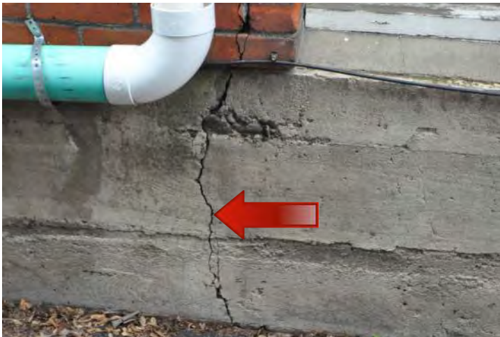
Figure 37: Similar to Figure 36, this crack in the concrete foundation located on the south side of the building, continues up through the brick to the top of the building. The crack is likely due to settlement of the foundation. Also note that the blue drain pipe is held by straps anchored directly into the brick units rather than into mortar joints. Locating anchors in mortar joints is less likely to damage the irreplaceable brick materials and is easier to repair in the future.
