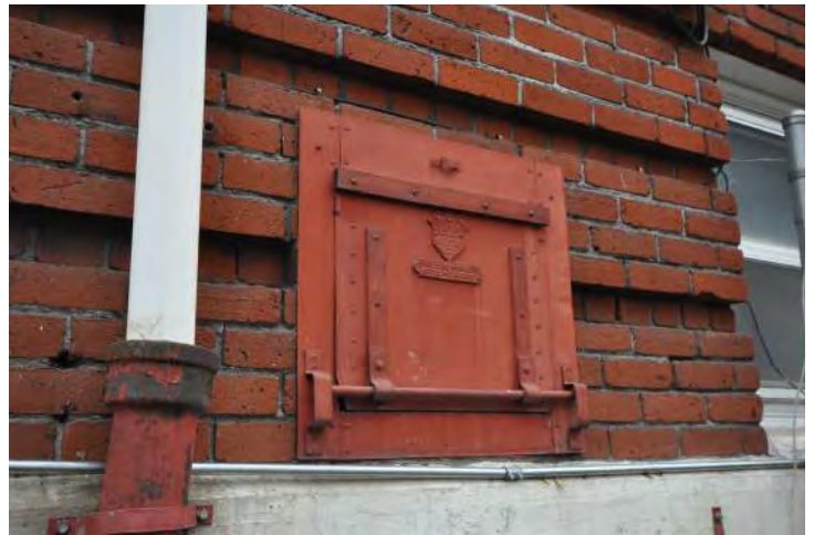
Figure 29: Detail at coal chute and downspout connection at the east elevation of the Library. Further investigation of the brick at the coal chute may help determine the original brick color and finish. The "open hub" connection between the schedule 10 PVC downspout and cast iron drain pipe may lead to areas of ice that can further damage the masonry wall systems due to freeze/thaw cycling.
