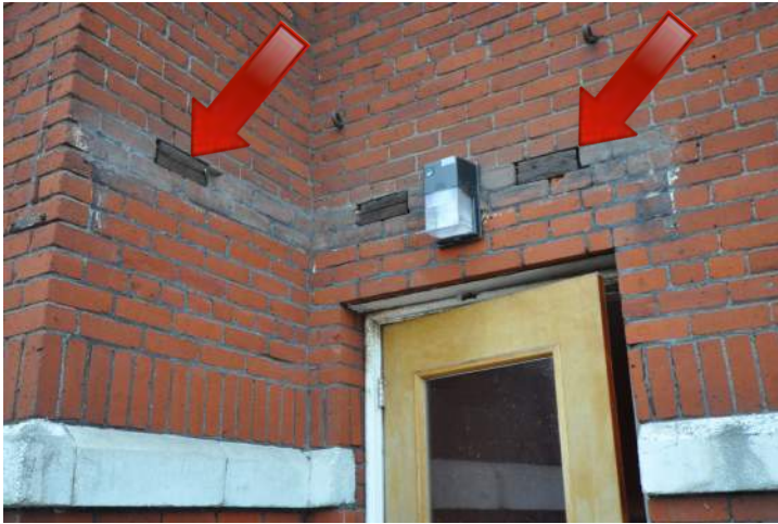
Figure 30: The wood blocking in the masonry wall at the exit door at the southwest corner of the building suggests that there may have been a canopy at this location at one time. The wood blocking may have been anchor points for the canopy framing. The remaining wood can absorb and hold increased moisture that can lead to insect habitation and infestation of the building. In addition, the higher level of moisture in the area can damage the masonry wall system through freeze thaw action. Removal of the wood and infilling the opening with in-kind masonry materials is recommended.
