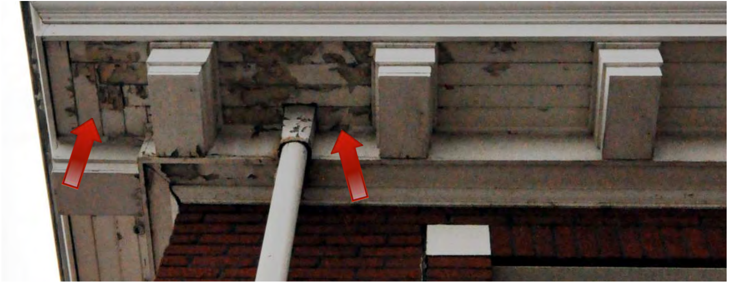
Figure 48: This downspout at the northeast corner of the building shows signs of significant and ongoing water leakage around the downspout. There is a high likelihood of rotting wood in addition to the observed paint damage at all downspouts on the building. The integral gutters and downspout connections should be immediately repaired to prevent further damage to the wood cornice and roof structure. © Richaven Architecture & Preservation, 2020. DSC_0033.JPG.
