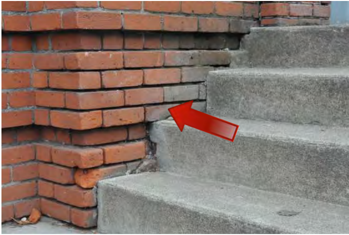
Figure 19: Mortar deterioration adjacent to the main entry stairs on the north elevation is severe and repointing is recommended. Mortar deterioration may have been caused by back splash of rainwater from the steps or application of ice melt products. Repair and protection of the brick and repointing of the mortar joints is highly recommended. In addition, it appears that the concrete stairs may have been installed after the brick walls were constructed due to the tothing of the concrete into the brick. This may result in added stresses on the brick walls and concrete stair structure, as observed in Figure 21.
