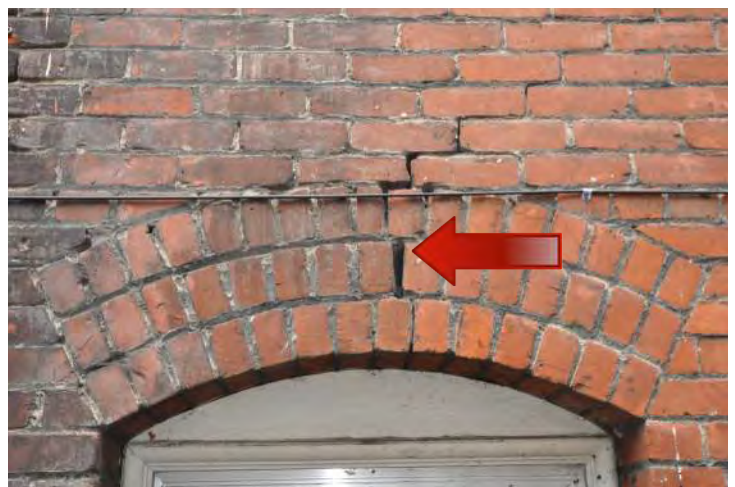
Figure 18: Detail at cracks in brick wall system, south elevation. © Richaven Architecture & Preservation, 2020. DSC_0056.JPG.
