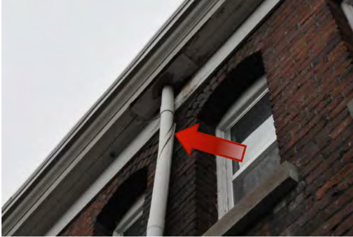
Figure 43: This downspout on the south side of the building shows significant damage, allowing stormwater to flow down the wall and saturate the masonry wall system. Immediate repairs to this downspout are recommended as well as repointing of the brick and wood repairs at the cornice and repair of the integral gutter to prevent leaking water into the building structure.
