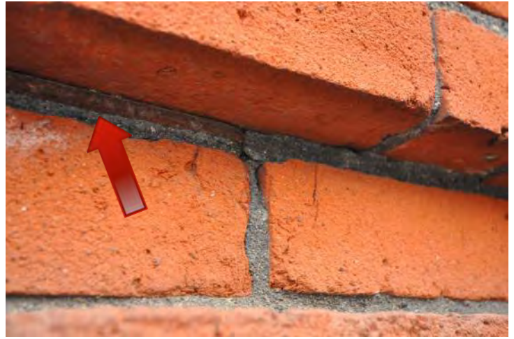
Figure 28: Detail at masonry wall system that was abrasively cleaned. This detail illustrates the porous core of the bricks that are exposed to the weather. Such exposure will likely lead to accelerated deterioration of the brick masonry due to freeze thaw cycling. Long term moisture saturation of the masonry wall system is also possible and may lead to disaggregation of the brick masonry units themselves. This detail also illustrated a steel lintel angle at the top joint in the recessed course. While exhibiting minimal corrosion, it is recommended that all exposed steel is painted to prevent corrosion where possible. However, corrosion due to high levels of moisture in the masonry wall system may also lead to accelerated corrosion of the steel building components.
