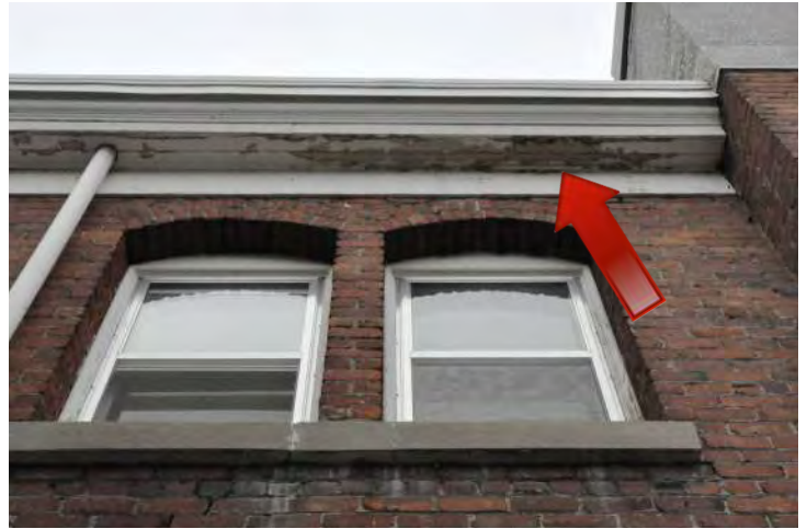
Figure 52: Extensive water damage on the underside of the cornice on the south elevation indicates that there is significant water leakage from the downspout running along the horizontal soffit boards.
