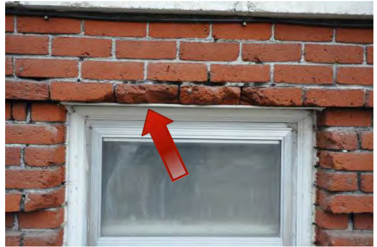
Figure 32: Detail at a basement level window at the east elevation of the Library. Severe damage to the masonry is observed due to the abrasive cleaning and likely mechanical/impact damage as well. The extent of damage at this window location make weatherproofing of the building difficult. Replacement of the damaged brick with matching in-kind materials and repointing of the joints in this area is recommended. In addition, the steel lintel angle at the head of the window is observed and is potentially exposed to the weather. Protection of the steel wall elements is recommended to prevent corrosion and rust jacking.
