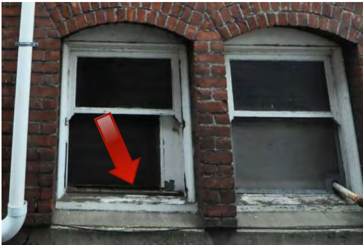
Figure 51: At this basement window on the south elevation of the building, deterioration of the paint finishes and glazing compound is observed. In addition, the bottom sashes of these two windows have been in-filled to allow for pipe and ventilation penetrations. These windows are immediately and fully repairable through consolidation of the wood materials, installing new glazing compound, and repainting of the windows.
