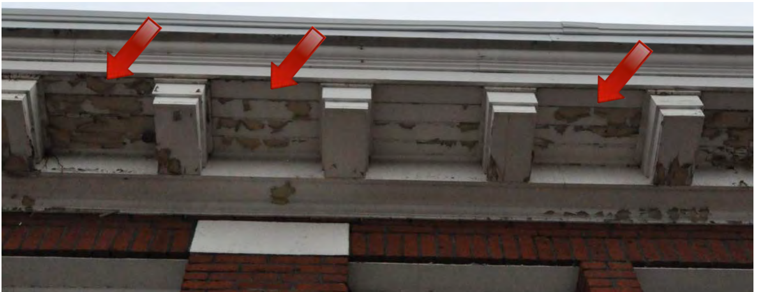
Figure 49: Peeling paint and wood damage at locations of the cornice away from the down spouts indicates that there may be additional leaks in the integral gutters, water traveling horizontally on the top of the soffit boards before soaking through to the paint coatings. Further investigation of the roof system and attic spaces is recommended to ascertain if water damage is more extensive than observed from the exterior. © Richaven Architecture & Preservation, 2020. DSC_0027.JPG.
