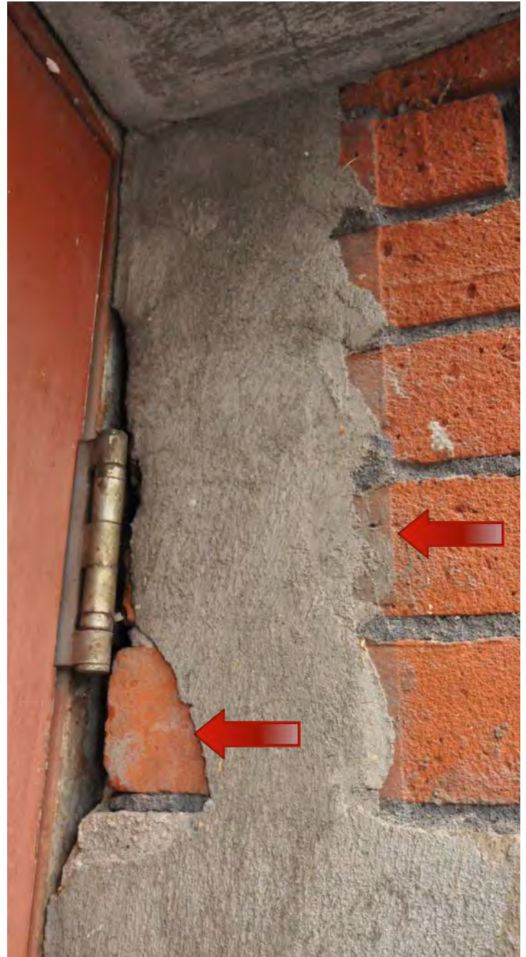
Figure 25: Masonry detail at the north side of the basement door on the east elevation of the Library. The brick masonry appears to have been protected by another material at the time the masonry was cleaned, as indicated by the vertical line between the smooth face of the masonry fire skin at the rough surface of the cleaned masonry. With reference to Figure 23, this detail suggests that the original color of the masonry was a traditional red colored fired brick. The amount of the brick removed in the abrasive cleaning process is also apparent. © Richaven Architecture & Preservation, 2020. DSC_0073.JPG.
