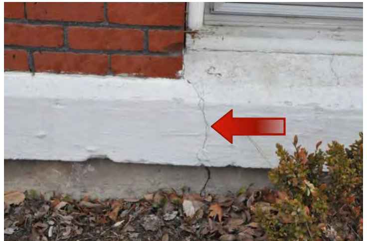
Figure 39: Similar to the two cracks in the precast concrete belt course in Figure 38, the crack through the foundation and the precast concrete course are the result of the vertical cracks telegraphing through this building element. Such cracks should be repaired to prevent water intrusion into the masonry wall system that promotes deterioration.
