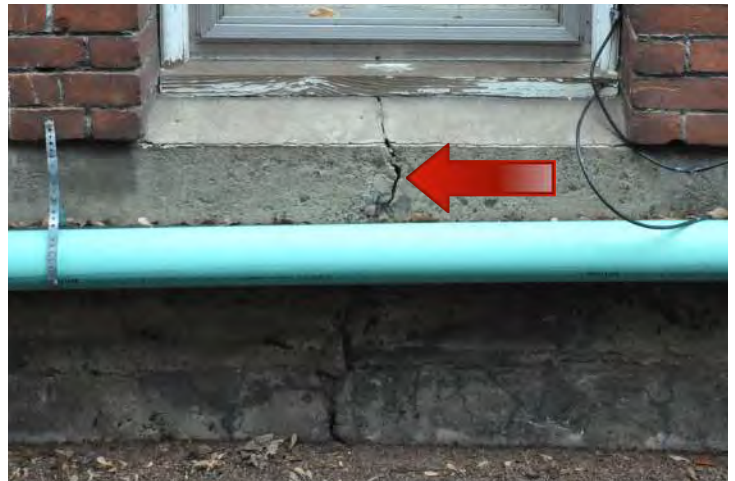
Figure 17: Detail at cracks and failed sealant repairs, south elevation. © Richaven Architecture & Preservation, 2020. DSC_0045.JPG.
