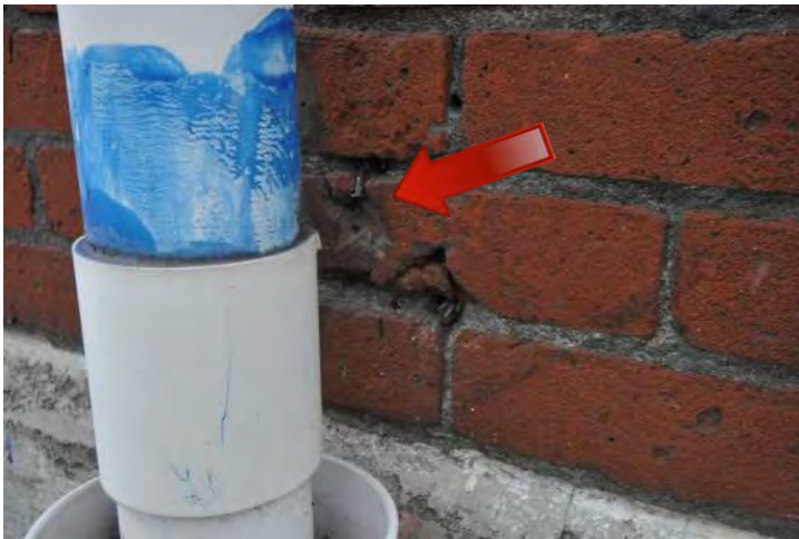
Figure 27: Masonry detail at a downspout on the south elevation of the Library. At this location, previously installed anchors remain in the masonry wall system and should be removed. In addition, it appears that other anchors have been removed and the masonry wall system has been damaged in the process. Repointing of the mortar joints and in-kind replacement of the brick is recommended.
