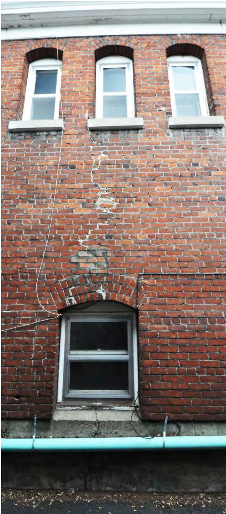
Figure 15: Full height crack in concrete and brick, south elevation. © Richaven Architecture & Preservation, 2020. DSC_0044.JPG.
