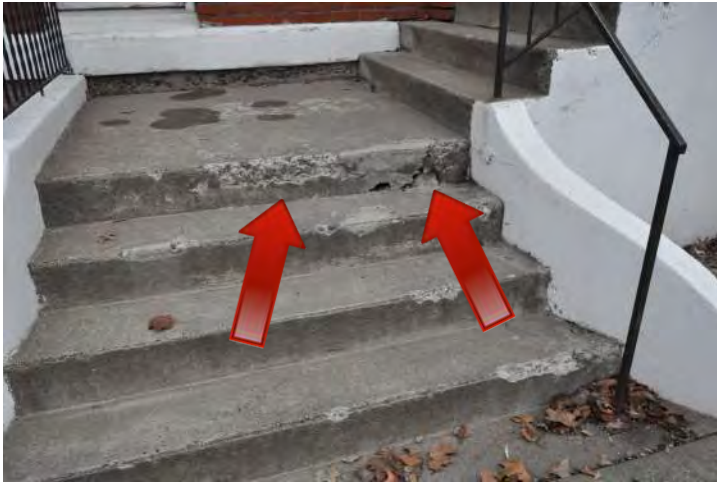
Figure 33: The concrete steps at the north main entry to the Library exhibit severe freeze/thaw damage likely due to ice melt chemicals applied to the steps. Repair of this type of damage may be possible through small localized patches or through removal of sections of the stairs and replacement in-kind. Use of ice melt products is not recommended for this type of area. Consider use of heat melting systems under the stair.
