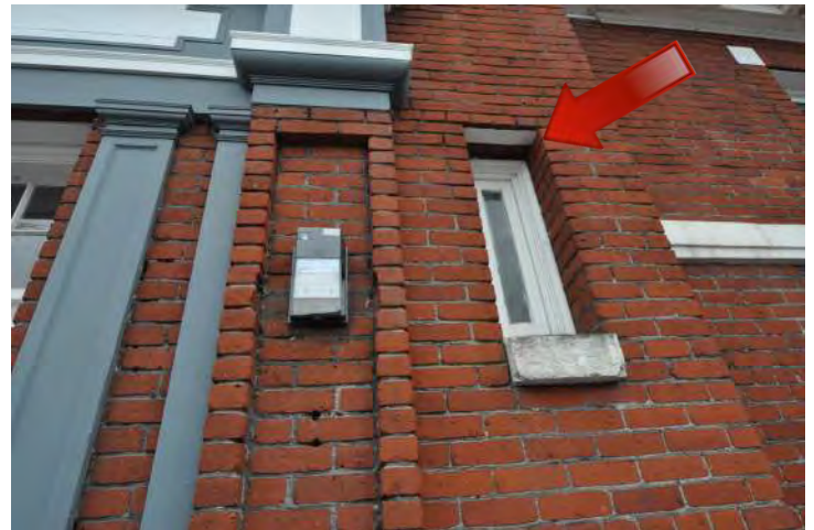
Figure 22: Masonry wall detail on the west side of the main north entry demonstrates deterioration similar to the east side. Additional noteworthy observations include the replacement light fixture which does not appear to be weatherproofed at the junction with the wall and the white-painted steel lintel at the head of the window. Steel lintels are observed at all window openings and appear to be in fair condition with minimal corrosion and rust jacking.
