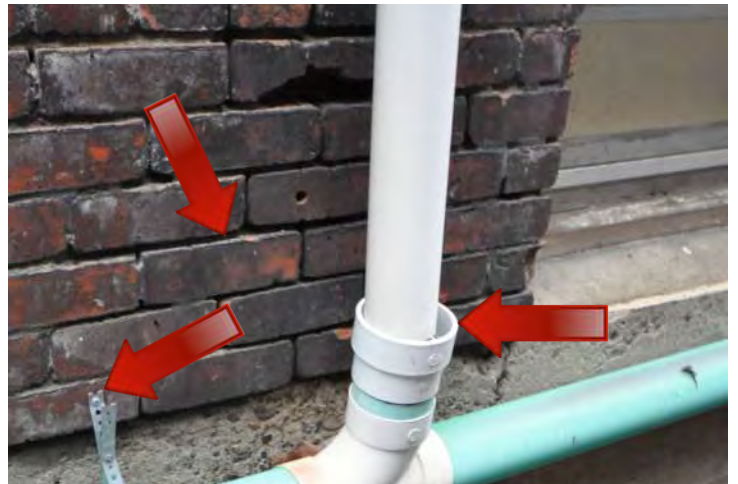
Figure 46: Continuing the downspout shown in Figure 43 and 45, this photo shows the "open hub" connection at the bottom which allows stormwater to splash out of the connection, erosion of the mortar in the brick joints, improper anchoring into the brick units, and significant soiling of the brick masonry (black staining).
