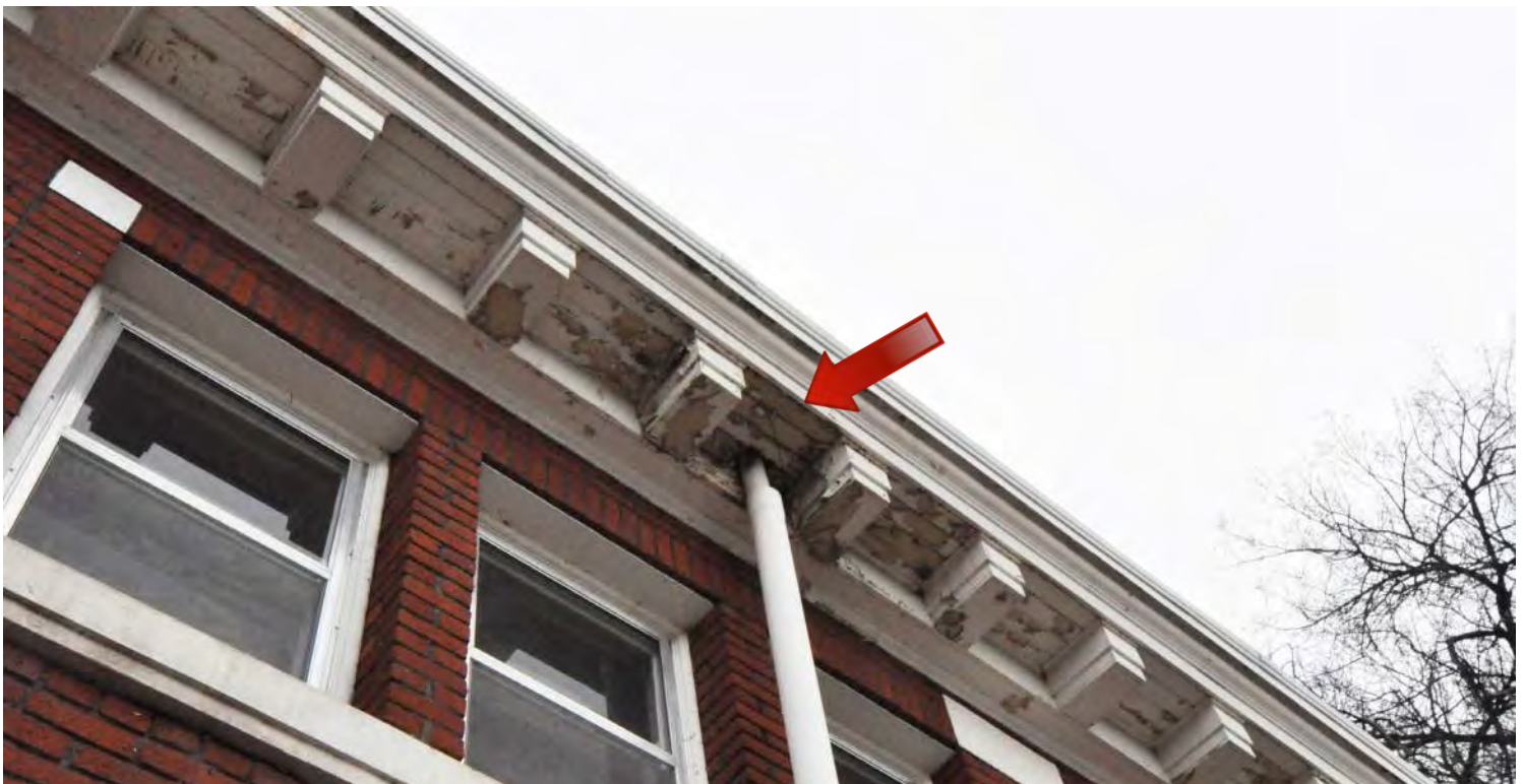
Figure 47: The painted wood cornice is damaged due to water leaking from the downspout connections due to blockage and freeze/thaw cycling. © Richaven Architecture & Preservation, 2020. DSC_0019.JPG.
