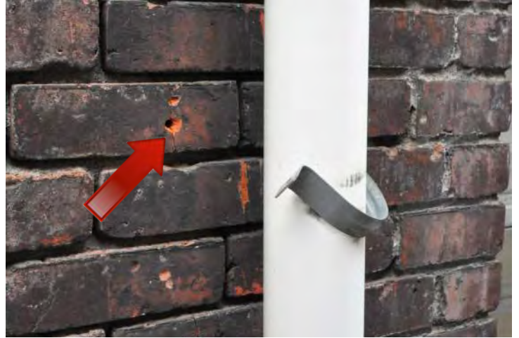
Figure 45: Continuing the pipe shown in Figure 43, this photo shows the erosion of the mortar into the masonry joints, as well as soiling and the missing strap anchor. Note also that the brick is cracked at the location of the anchor, compromising its integrity and reducing the structural integrity of the wall.
