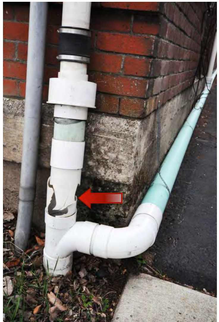
Figure 40: A vertical downspout at the southwest corner of the building is shattered due to freeze/thaw cycling abetted by debris in the pipe. © Richaven Architecture & Preservation, 2020. DSC_0037.JPG.
