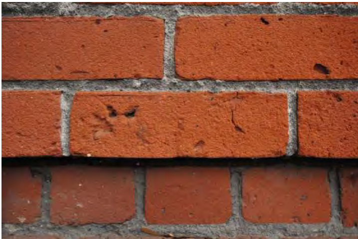
Figure 24: Masonry detail at the east elevation of the Library reveals that the abrasive cleaning of the wall has exposed pockets in the masonry as well as the grog used in the manufacture of the brick. The mortar is also observed to be rough and the tooling of the joint worn away by the cleaning potentially making it subject to more rapid deterioration. Light cleaning, sealing and coating with anti-graffiti coatings should be considered to preserve the masonry wall systems. © Richaven Architecture & Preservation, 2020. DSC_0076.JPG.
