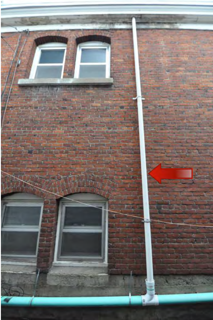
Figure 41: Typical of the drain pipes on the building, this vertical downspout on the south elevation has an "open hub" connection, light weight PVC piping, straps anchored directly into the brick, and there are signs of water related damage at the cornice.
