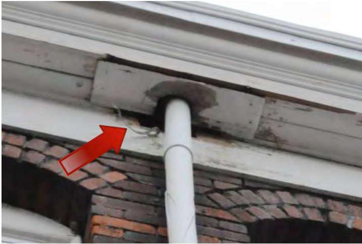
Figure 50: Severe damage to the cornice is observed at the downspout on the south elevation. Damage is so severe that an additional board has been installed to cover the opening. Note that the strap holding the downspout in place is broken and the downspout itself is shattered at this location. Eroded mortar at the brick joints due to the water saturation is also observed at this location.
