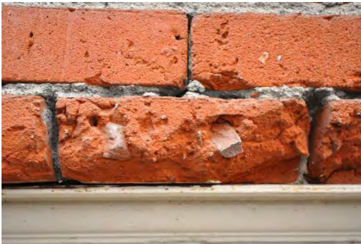
Figure 31: Detail at masonry wall system that was abrasively cleaned. This detail illustrates the porous core of the bricks that are exposed to the weather. Such exposure will likely lead to accelerated deterioration of the brick masonry due to freeze thaw cycling. Long term moisture saturation of the masonry wall system is also possible and may lead to disaggregation of the brick masonry units themselves. This detail also illustrated a steel lintel angle at the top joint in the recessed course. While exhibiting minimal corrosion, it is recommended that all exposed steel is painted to prevent corrosion where possible. However, corrosion due to high levels of moisture in the masonry wall system may also lead to accelerated corrosion of the steel building components.
