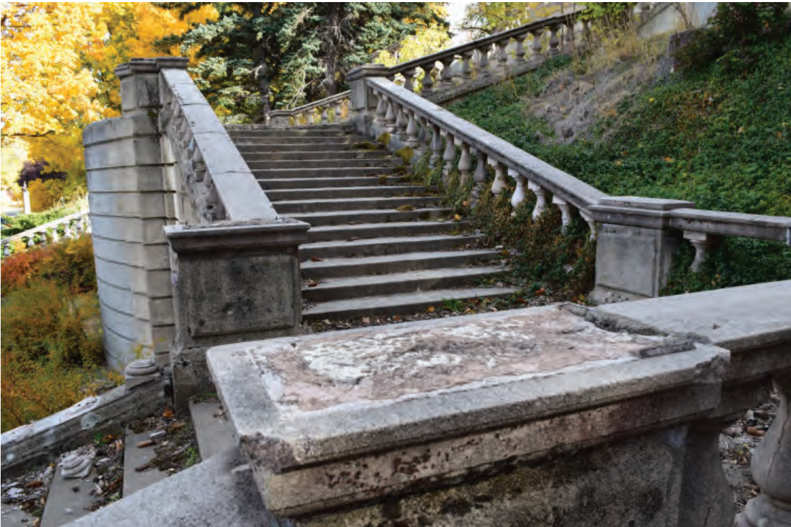
2. Grand Staircase west staircase entrance, facing east. Notice missing balustrade, encroaching vegetation, missing detail on balustrade post, and leaning of retaining wall.. 10/19/2021.
