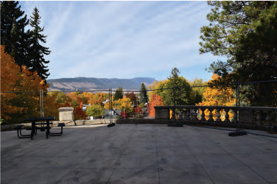
6. Top landing, facing north. Notice missing balustrade and temporary safety fencing. 10/19/2021.
