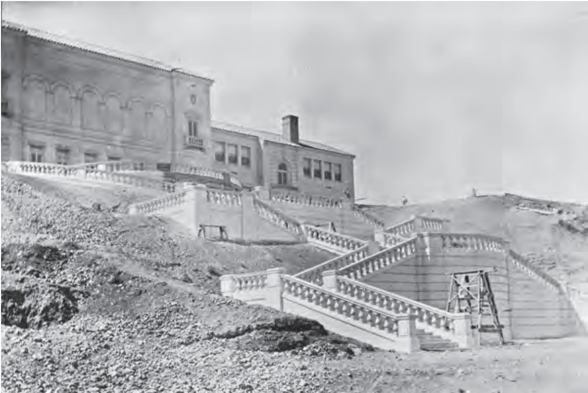
9. Grand Staircase under construction, 1927/28. Northeast corner, facing southwest. Courtesy of Eastern Oregon University Digital Archives.
