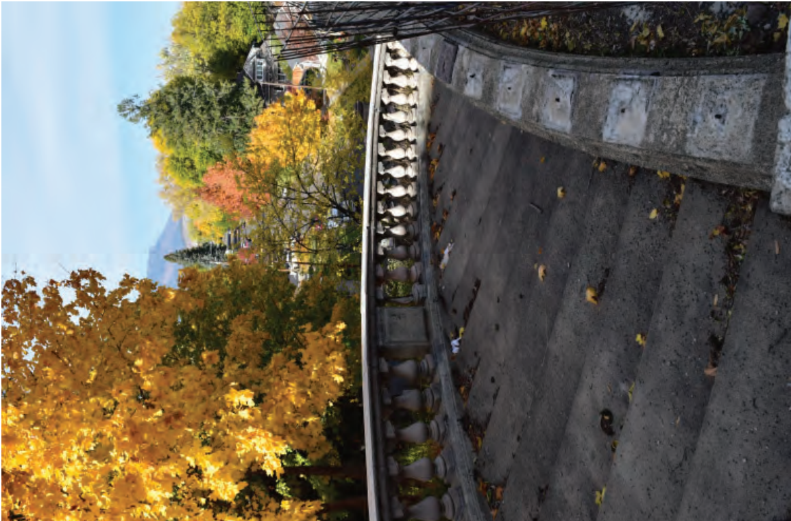
5. Photo taken from west stairway descending from top landing, facing north. Notice missing balustrade. 10/19/2021.
