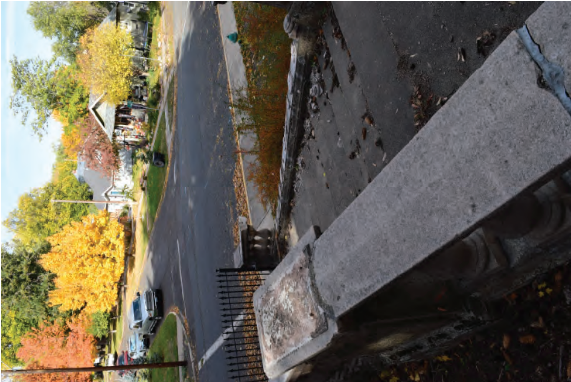
3. Grand Staircase west staircase entrance, facing north. Notice missing balustrade, missing detail on balustrade post, and safety fencing. 10/19/2021.
