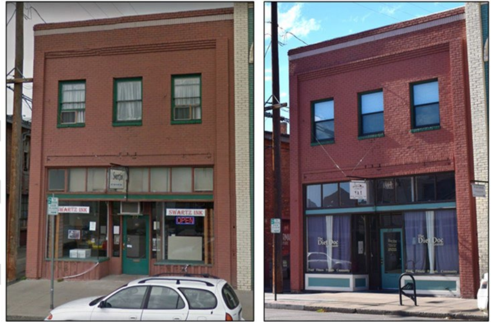
212 Fir Street is a good example of a rehabilitated storefront. Note the new paneled bulkhead beneath the storefront windows. (Source for image on left.)
